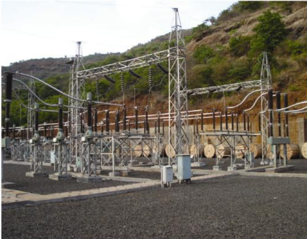
2x 25 MVA, 110 KV Switch Yard, Sub Station At Lavasa
